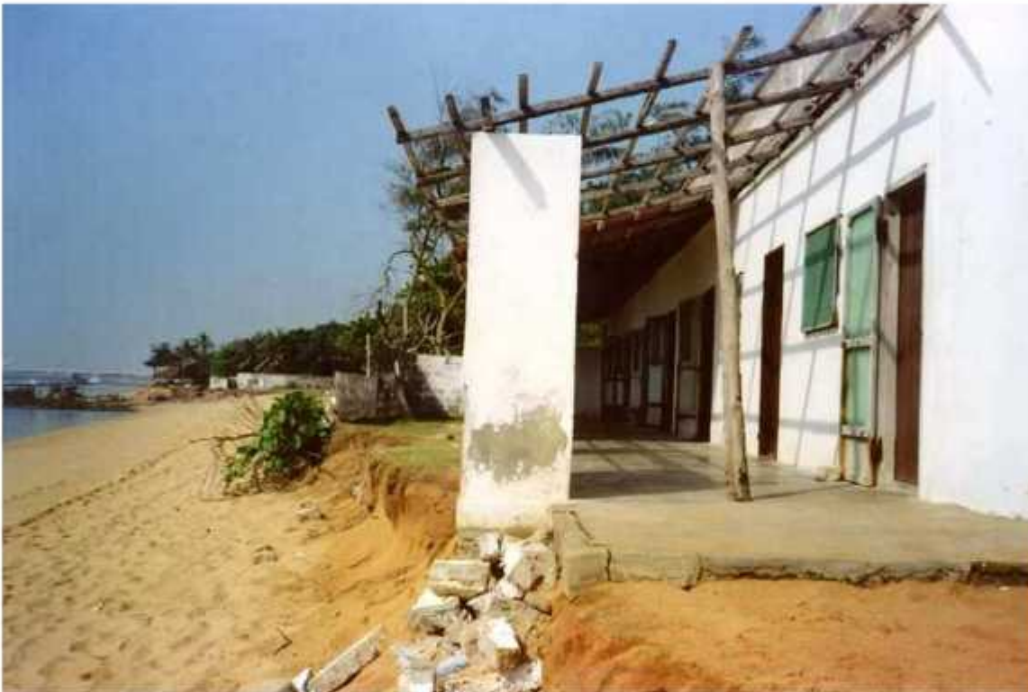
Figure 4: Beach affected by coastal erosion at the Ramatou Hotel (east of PAL) in November 2003
